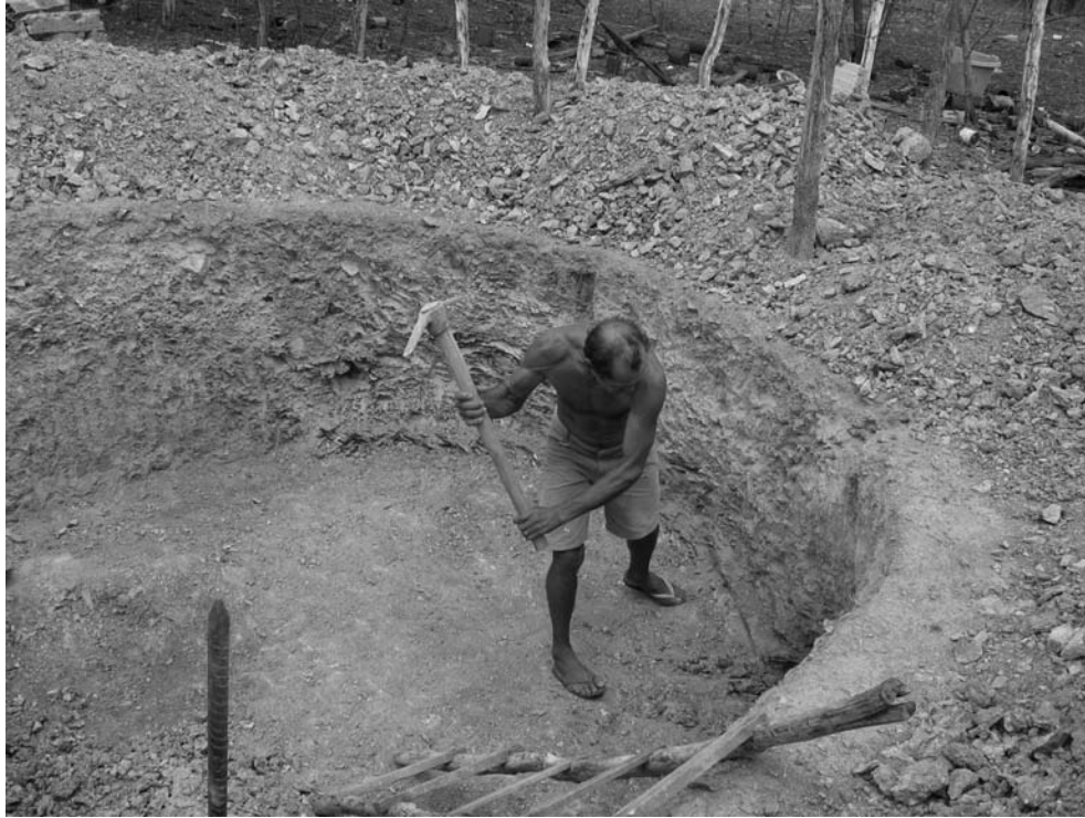
FIGURE 7. Carving out space for a new cistern for rainwater capture and storage.
